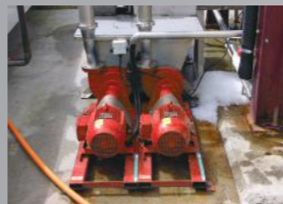
Horizontal Pumps at Chicken processing facility
