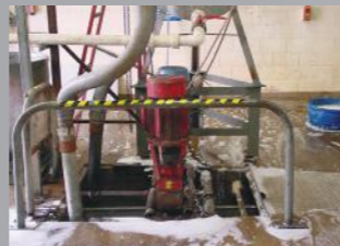
Volume Pump at Meat processing facility
